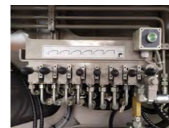
Direct Boom control emergency panel
